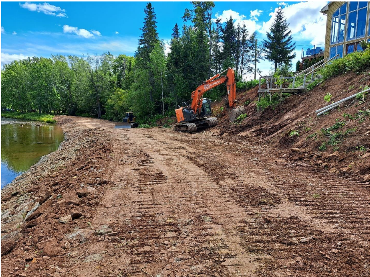
Figure 29: 2022 Project undertaken by private landowner to protect their house on a failing riverbank
