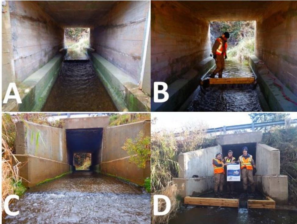
Figure 33: C-011 A) before baffle; B) after baffle; C) before chute; D) after chute installation
