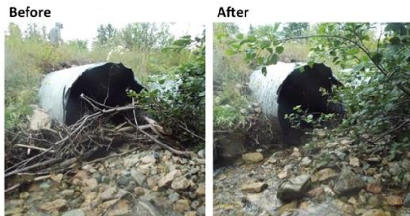
Figure 31: Before and after photos of C-022, located where Church Hill Road crosses Sheffer Brook
