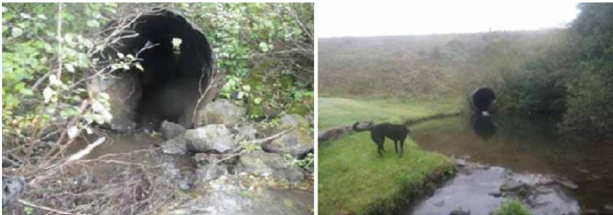
Figure 16: Route 126 culvert in 2012: collapsing inflow left, and perched outflow right.
