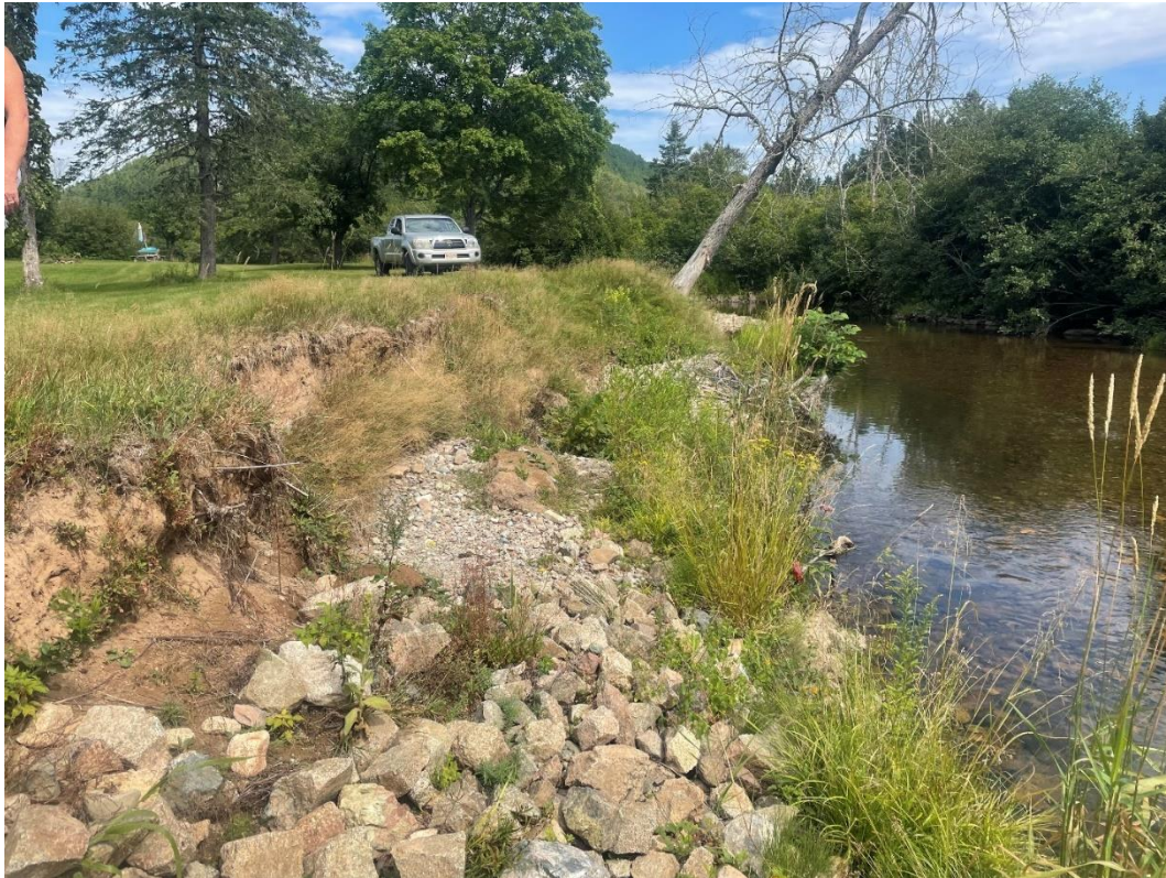
Figure 37: Looking downstream along the failing bank at the 2023 project
