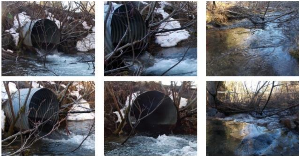
Figure 31: Plunge pool at C-051 before (top row) and after (bottom row) rock weir construction
