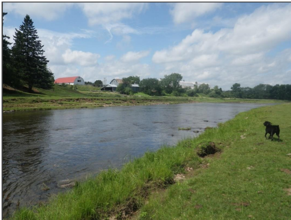
Figure 4: Failing banks on both sides of the river due to unrestricted access by dairy herd
