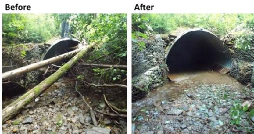
Figure 32: Before and after photos of C-041, where a logging road crosses Popple Intervale Brook.
