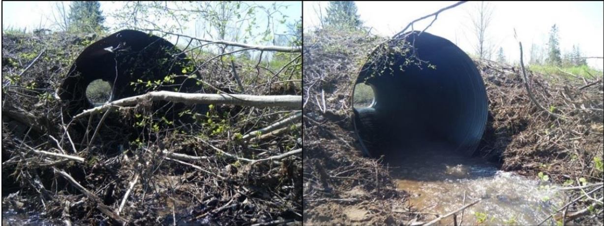
Figure 4.3 Culvert C-151 before and after PWA removed debris to make it passible in 2017
