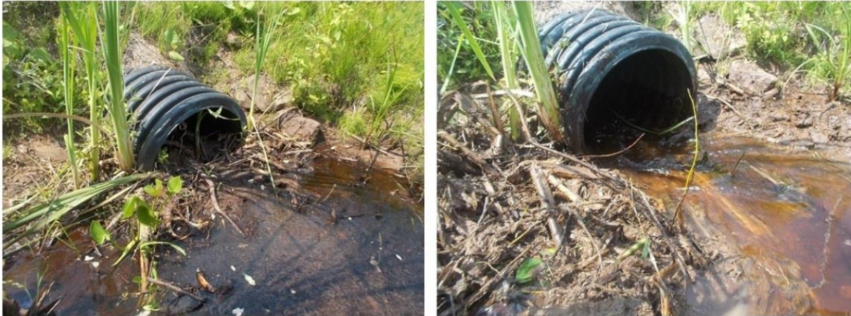
Figure 4.6 Culvert C-224 before and after PWA removed debris to make it passible in 2017
