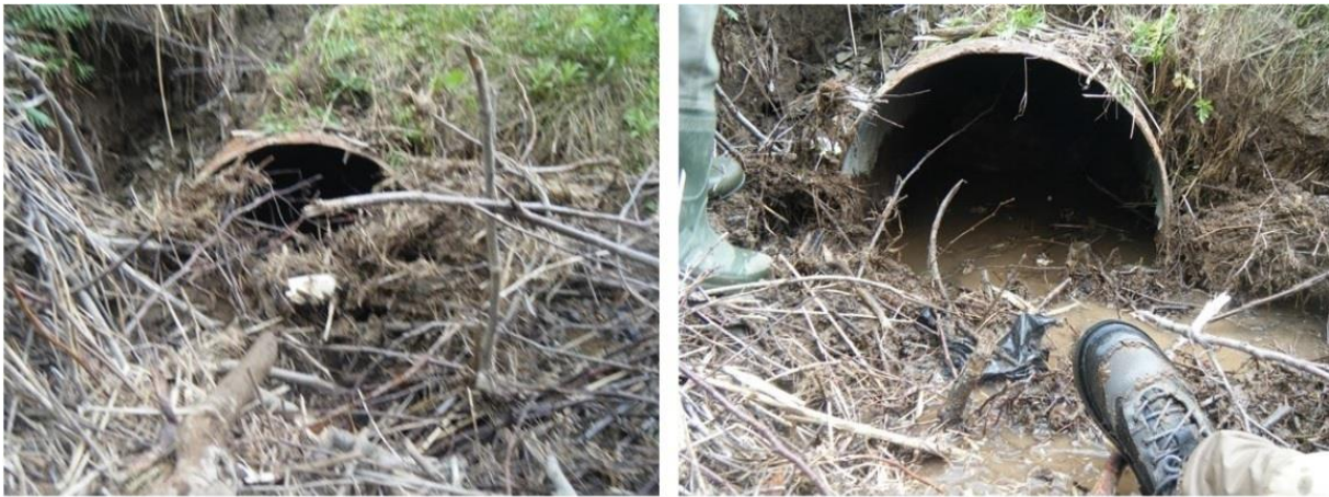
Figure 4.4 Culvert C-154 before and after PWA removed debris to make it passible in 2017
